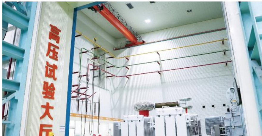
High-voltage Test Hall
